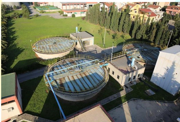
Example of Sewage Disposal Tuzla/Istanbul Municipality
