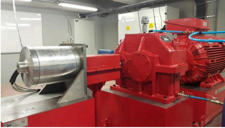
Electric Motor Test Bench Nominal Power 150 kW Nominal Torque 400 Nm (Garaj)
